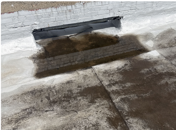
Ponding at the scupper with sediment staining
