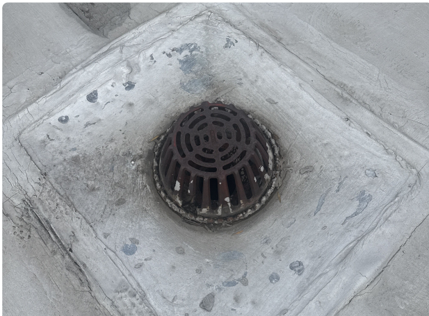
Exposed lead flashing at drain — new target patch required
