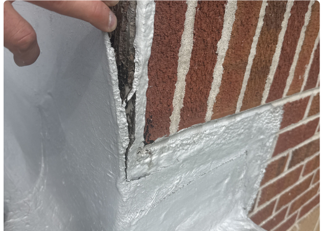
Open wall flashing at brick inside corner — direct water entry path
