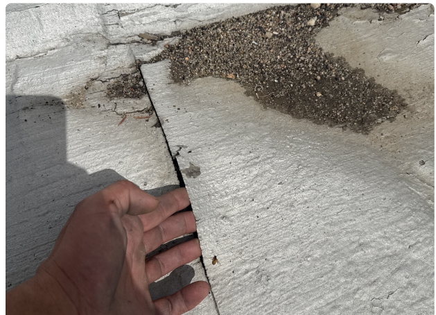
Field seam beginning to fail at the parapet base
