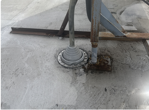
Metal-roof-type boot used on modified bitumen — wrong product; insulation soft underfoot in this area
