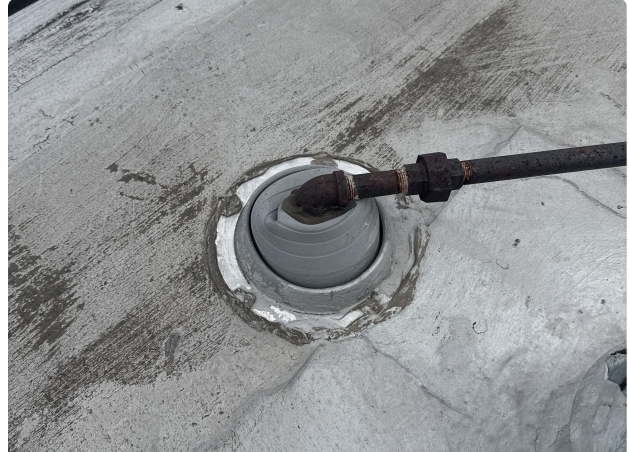
Pipe boot at gas line — pitch pan required
