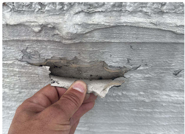
Coating peeling from wall flashing, exposing EPDM used as wall flashing on a modified bitumen roof
