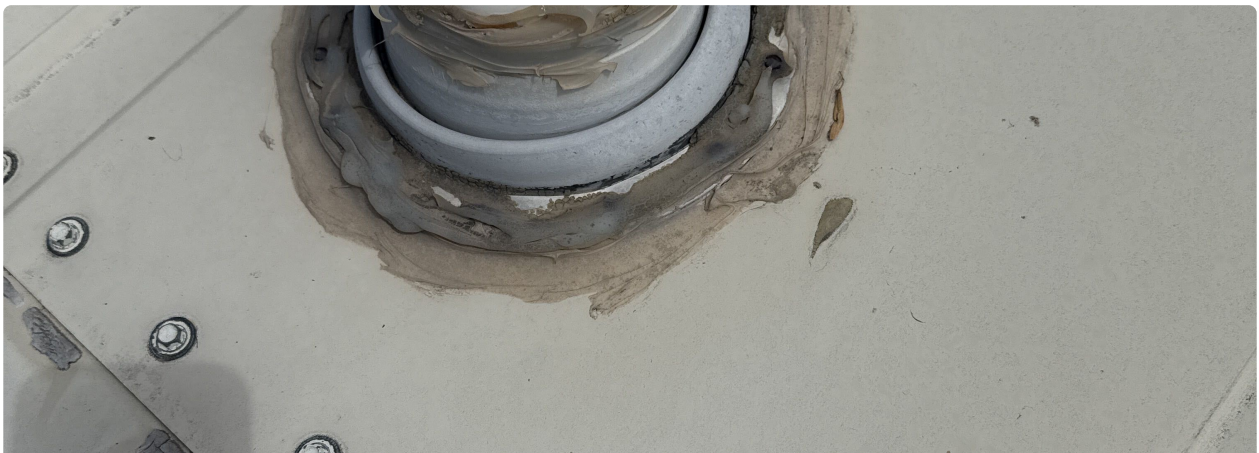
Pipe boot 3 — same condition
