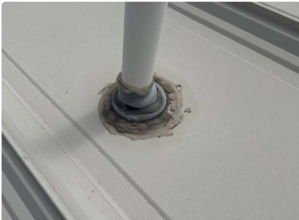
Pipe boot 1 — collar cracked, dried and smeared sealant, no positive seal
