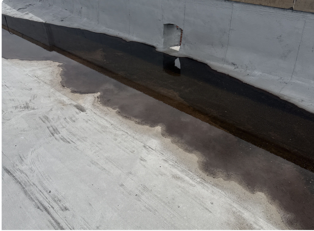
Ponding running the full length of the parapet toward the scupper
