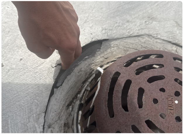
Open target patch at drain; rusted cast-iron drain, debris in sump
