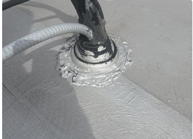
Rubber boot on conduit penetration — incorrect detail, pitch pan required
