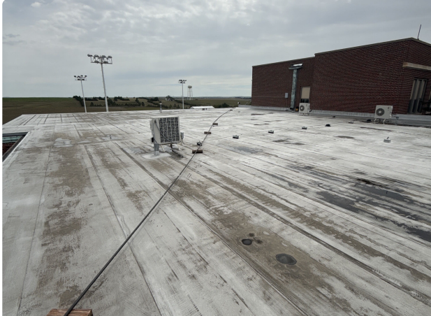
North section overview — coating heavily weathered, ponding areas, mini-split condensers on stands
