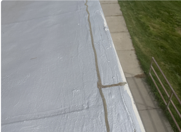
Silicone caulking at perimeter/edge termination — incompatible with this roof system
