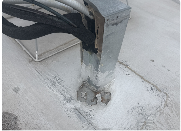
Sheet-metal conduit chase at HVAC unit — cannot be sealed; remove and install pitch pan
