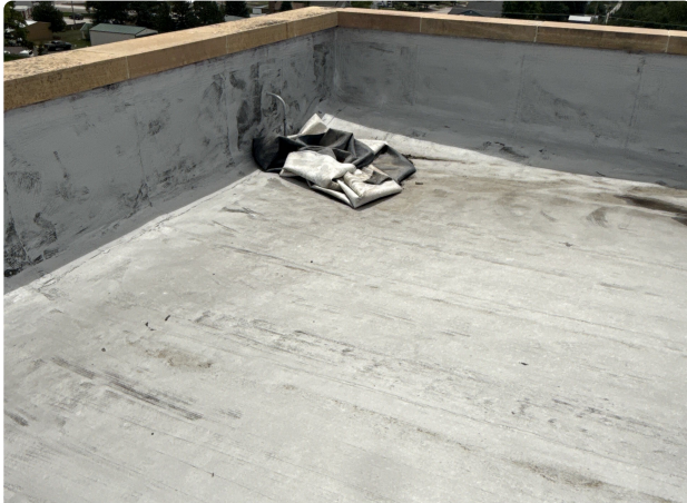
Loose membrane wadded in the corner — debris and wind hazard
