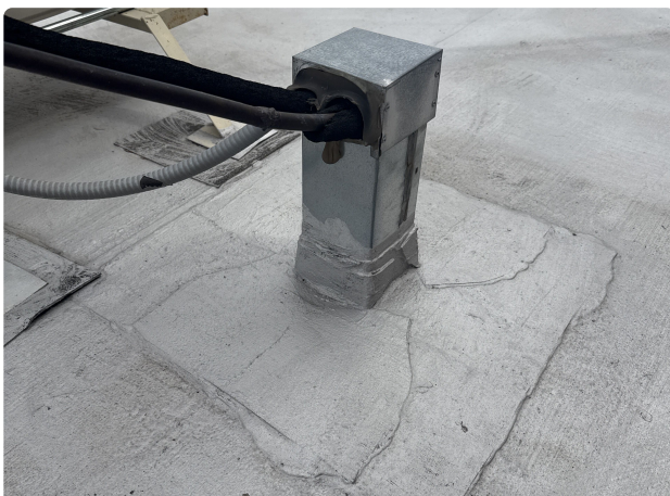
Fourth conduit chase at mini-split condenser — patch edges lifting
