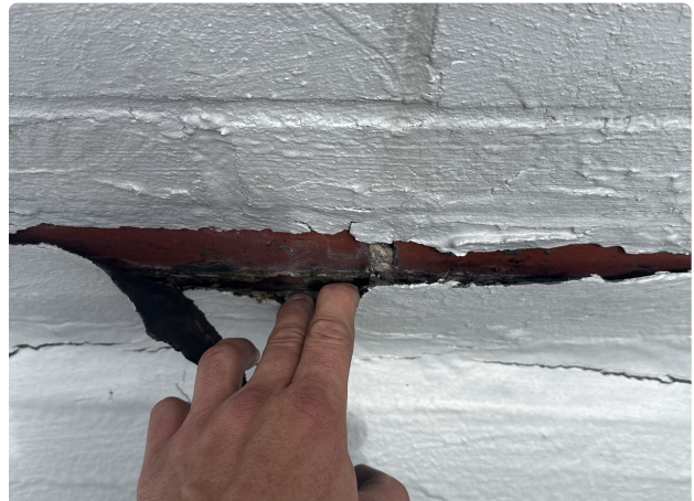
Wall flashing opening at parapet — gap wide enough to insert fingers
