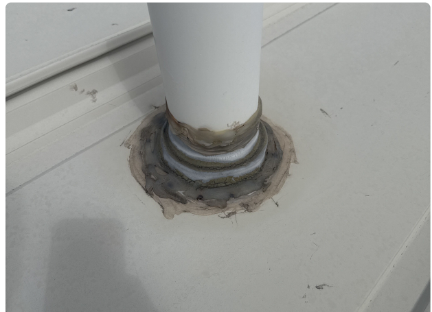
Pipe boot 2 — same condition
