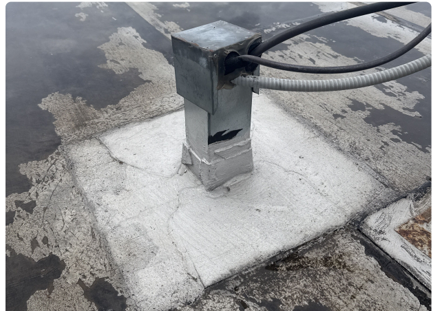
Third conduit chase; surrounding coating weathered and peeled, ponding water
