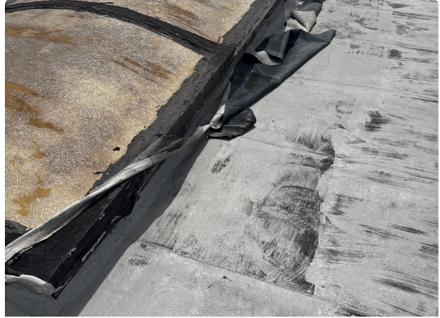
Loose EPDM sheet — prior temporary skylight cover, blown off into the parapet corner
