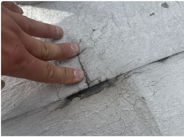
Base tie-in seam pushes water out underfoot — moisture in the system
