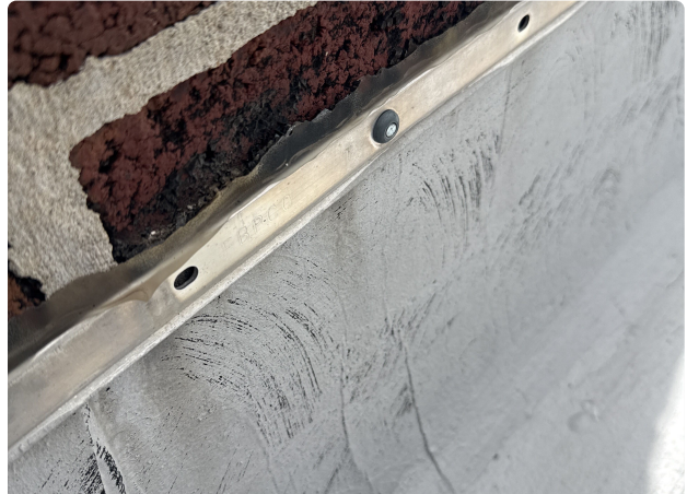
Termination bar sealed with silicone — incompatible
