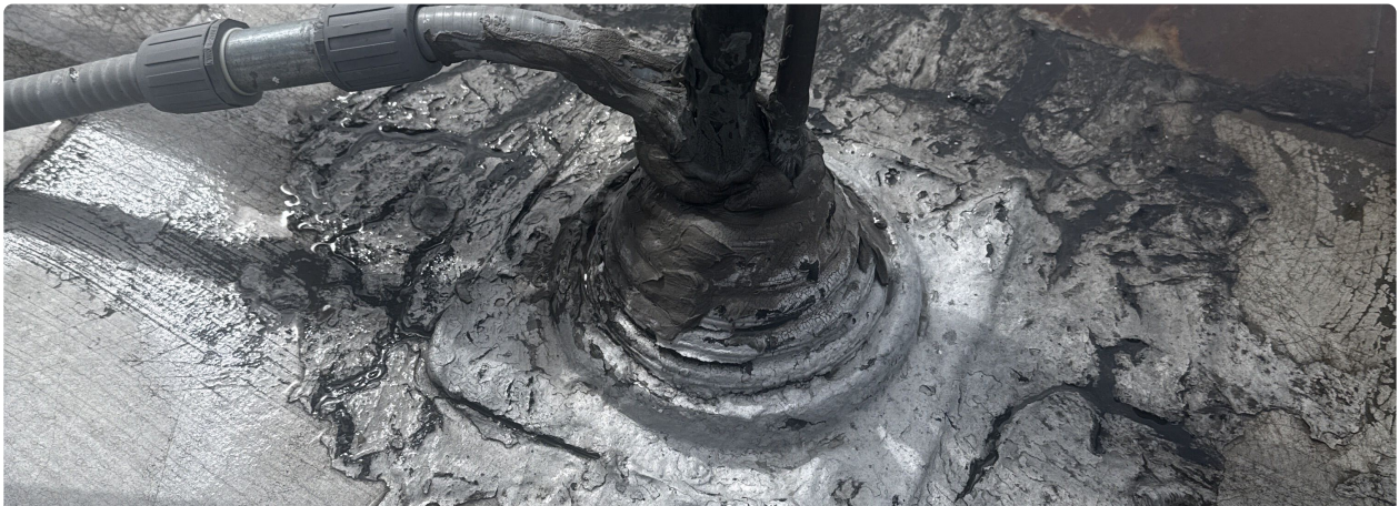
Second rubber boot at conduit penetration — pitch pan required
